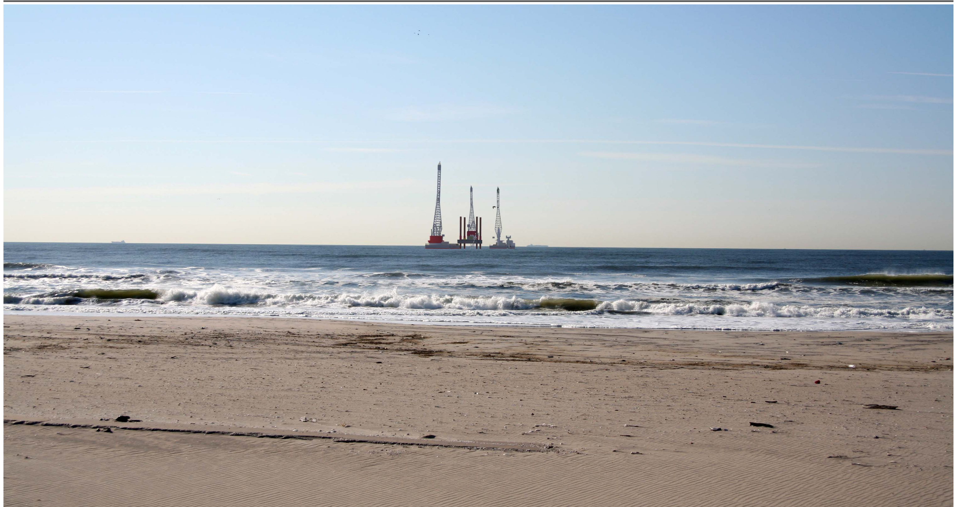
Simulated View - Drilling Operation and Pipe Laying Barge (near Exit Pit Location)
